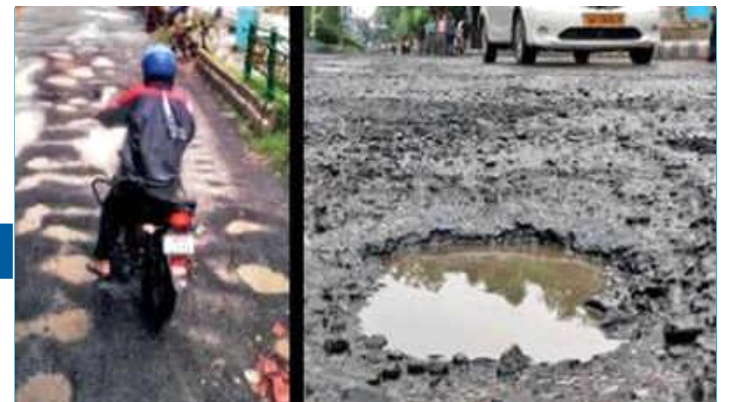
Deterioration of road and potholes
