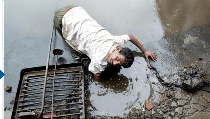
Blockages in Sewage lines
